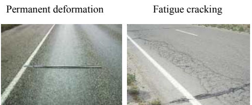
Fig. 2. Common distresses in asphalt pavements Reference [12].
