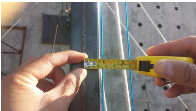
Image XXI. Plastic deformation outside the plane (residual) of one inch in average as a result of the total discharge of the structural system. (5).
